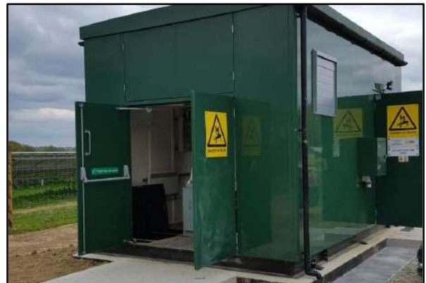
Example Transformer Unit on site
